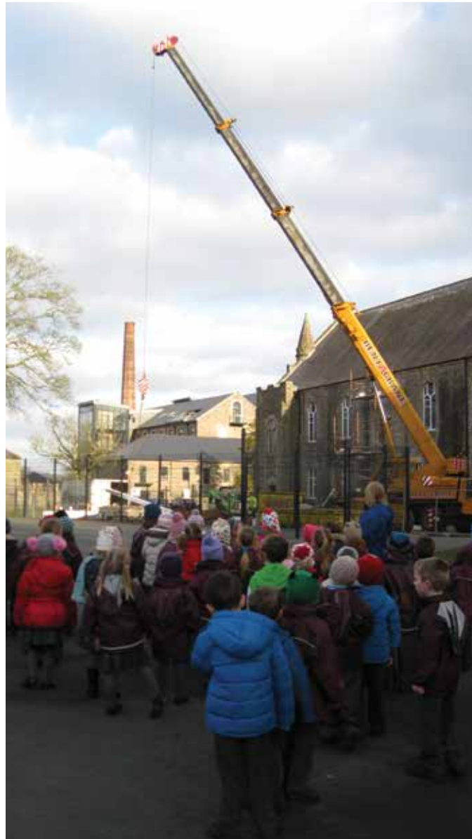
Primary 1 children re-visit their Hall to see the crane lifting the new steel structure which will hold the lift into place.
